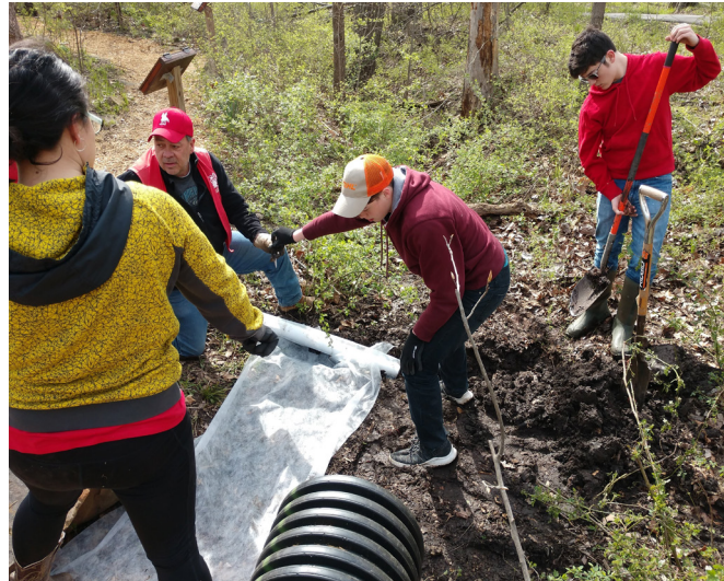
Jonathan Staten (15) and Daniel Gonzalez (14) work on improving drainage on the culvert at Deanna Rose Farmstead for their Science Matters project.
